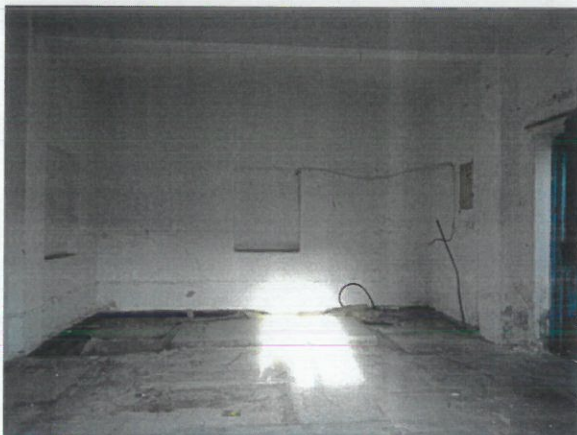
Interior statie pompare C8
