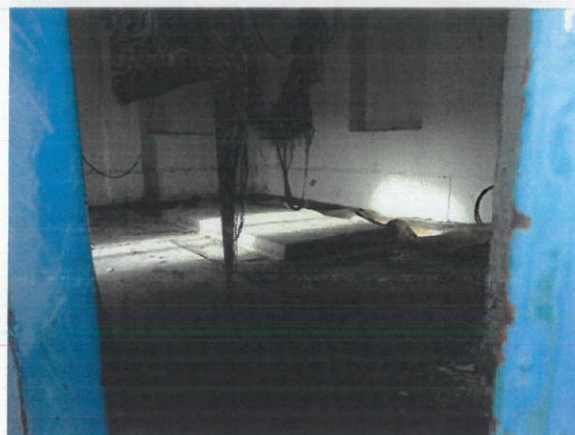
Interior statie pompare C8
