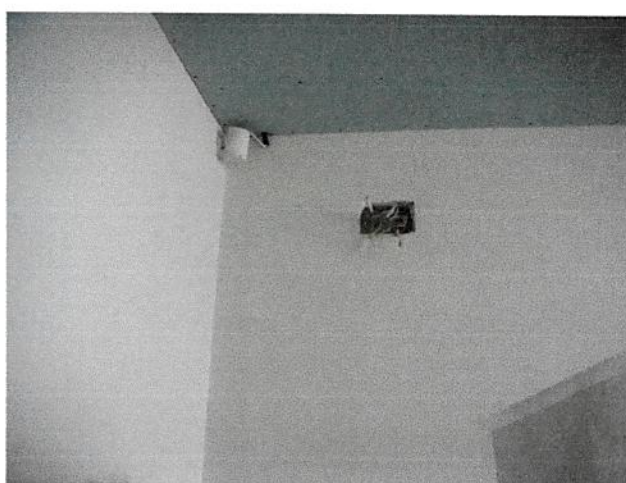
interior parter- instalatie alarma
